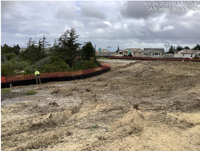
Cleared last of the trees and vegetation adjacent to Marina Heights and Abrams
